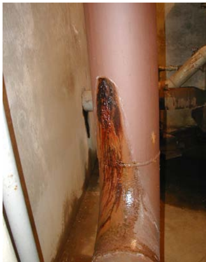
30 year old corroded pipe at Mixsawbah Hatchery
